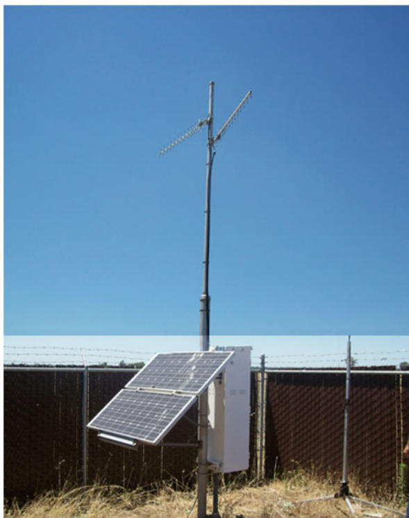
Fig. 6.3 GNSS CORS power supply and telemetry
