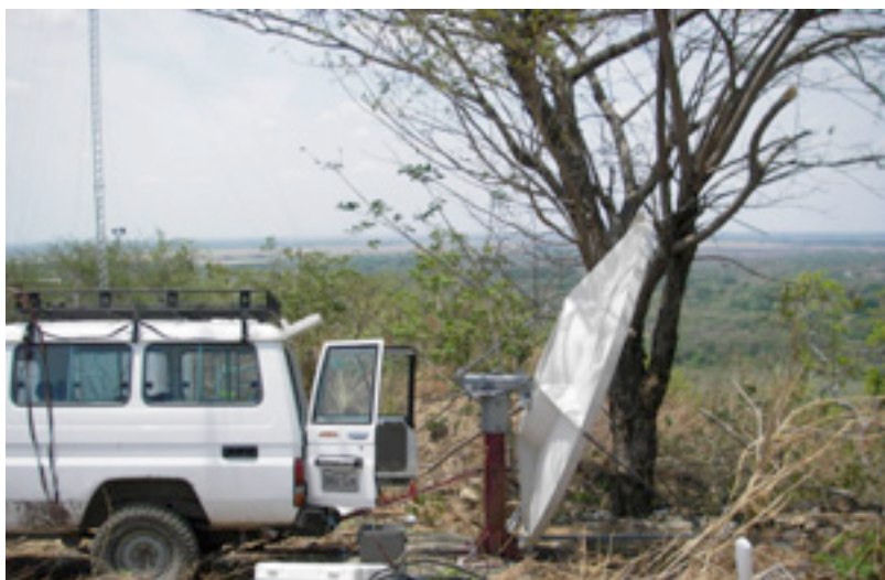
Figure 11.34: El Baúl antenna installation. Actual elevation was 1^\circ upward, since the antenna has an offset of 22.5^\circ .
