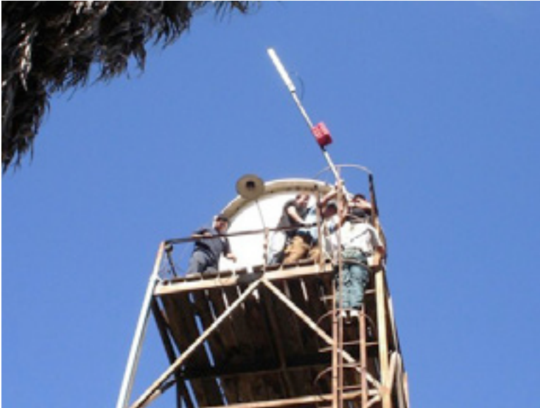
Figure 11.24: Implementation of node over a water tower in Batuco, Metropolitan Region, providing backhaul to Cabrati telecenter.
