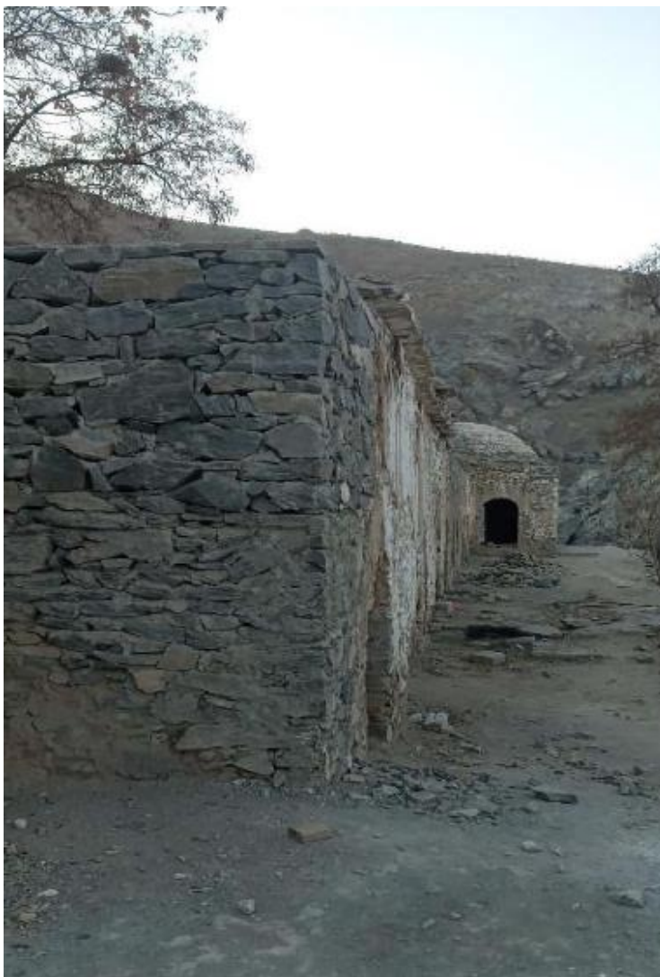
Front elevation Pictures of the Buddhist temple after renovation from the east
