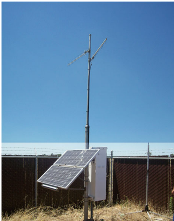
Fig. 6.3 GNSS CORS power supply and telemetry
