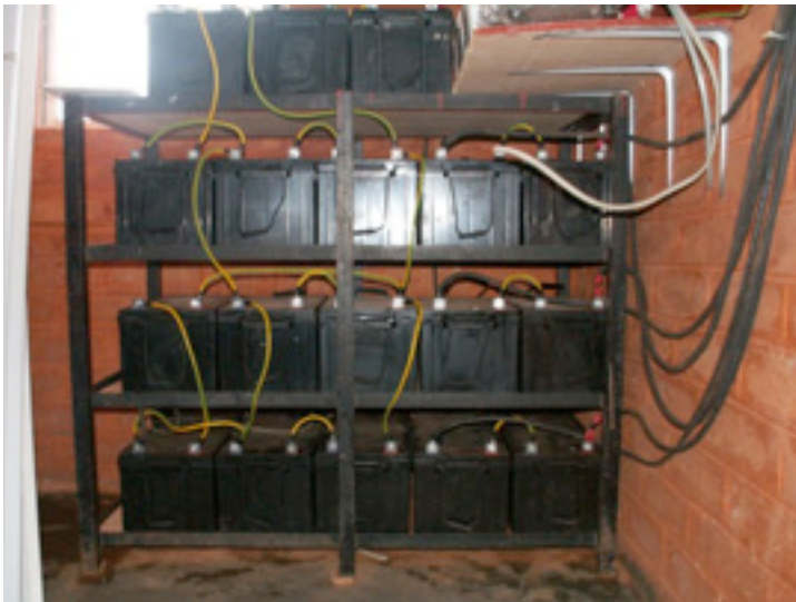
Figure 7.9: A battery bank of 3600 Ah, currents reach levels of 45 A during charging
