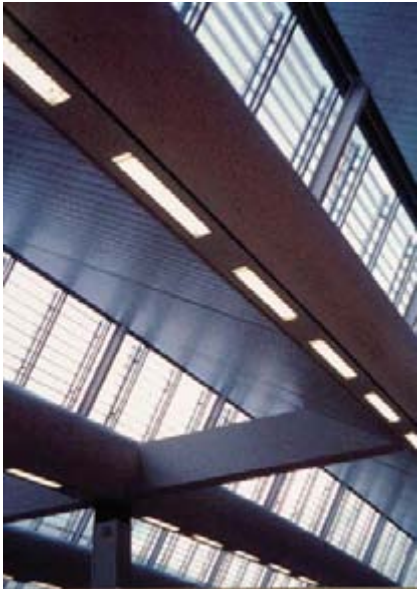
Detail of roof lighting
