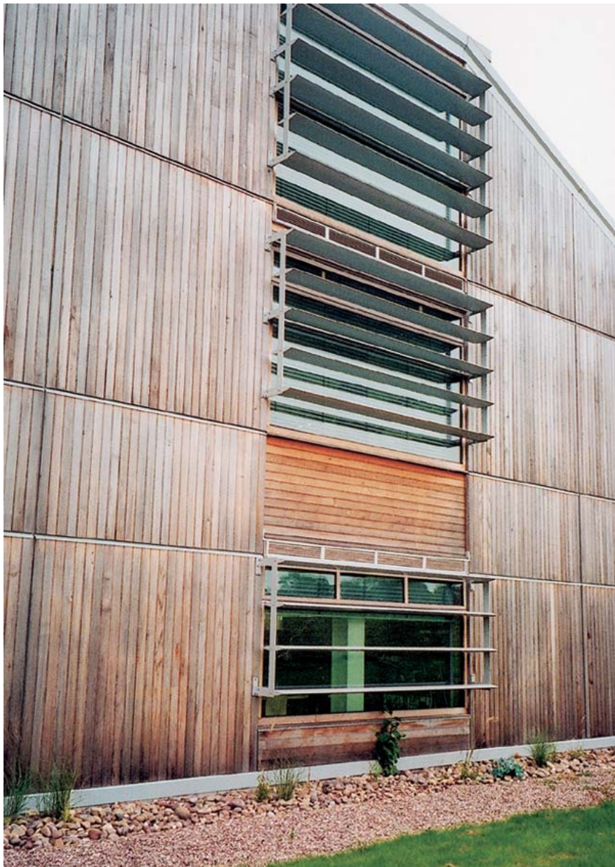
Exterior to show the application of reduced glazing and fixed louvers to southerly elevations
